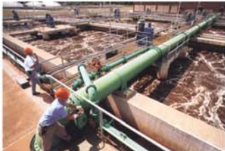
Waste water Treatment
